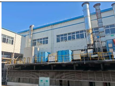
两级活性炭 (TA014) + 14#废气排气筒 (DA014)
