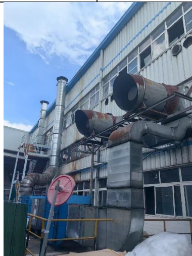
两级活性炭 (TA010) + 10#废气排气筒 (DA010)
