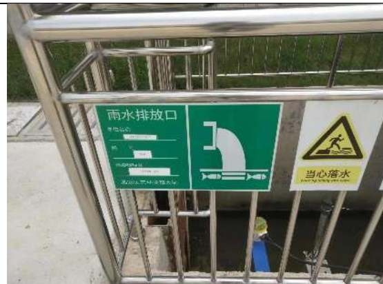
雨水排放口切断闸阀
