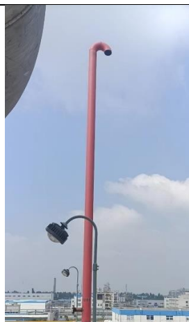
DA007 排气筒 (26m)
