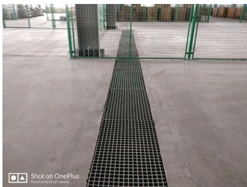
厂区冲洗水收集沟
